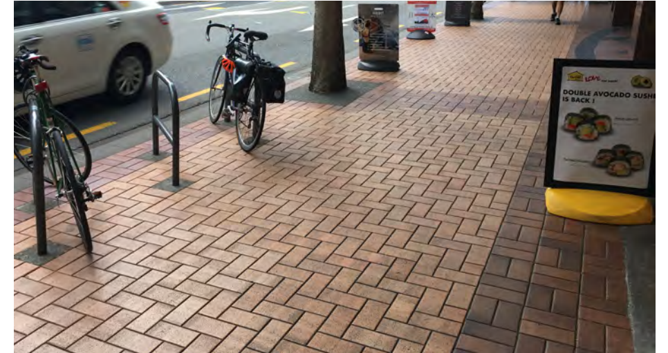
Paving on Willis Street is generally in good condition. Kerbs have a large format profile that lifts the sense of quality.
