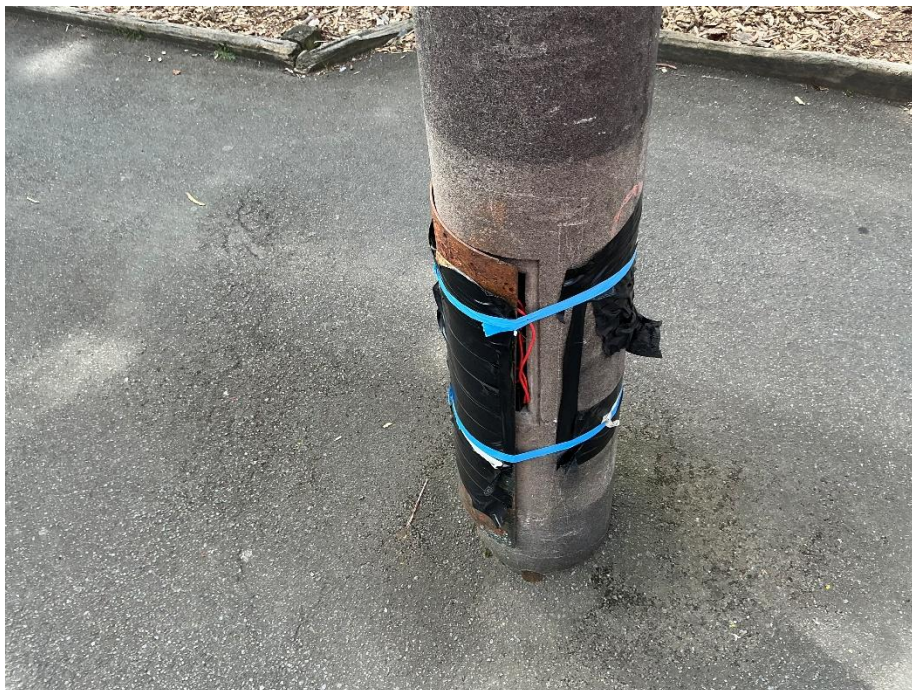
Figure 5-10: View of loose wiring at base of light pole
